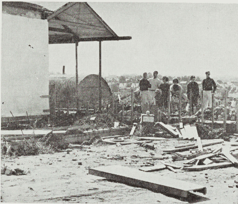
Several students survey the beginnings of the new auditorium which is being added on to the anxiously awaited College Union Building. The completion date is set for sometime early next year.
